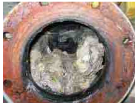
This is NOT what you want to see in your valve. Solids were getting trapped in the valve and clogging up the pipeline.
