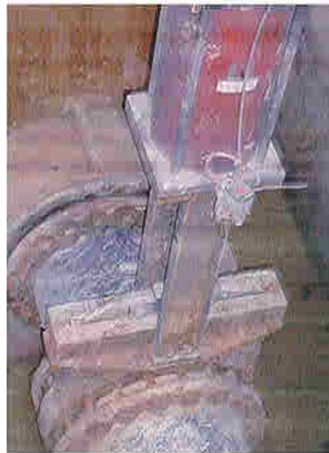
Two large-diameter valves from Red Valve will protect against overflow for the remainder of the dam's useful life.
