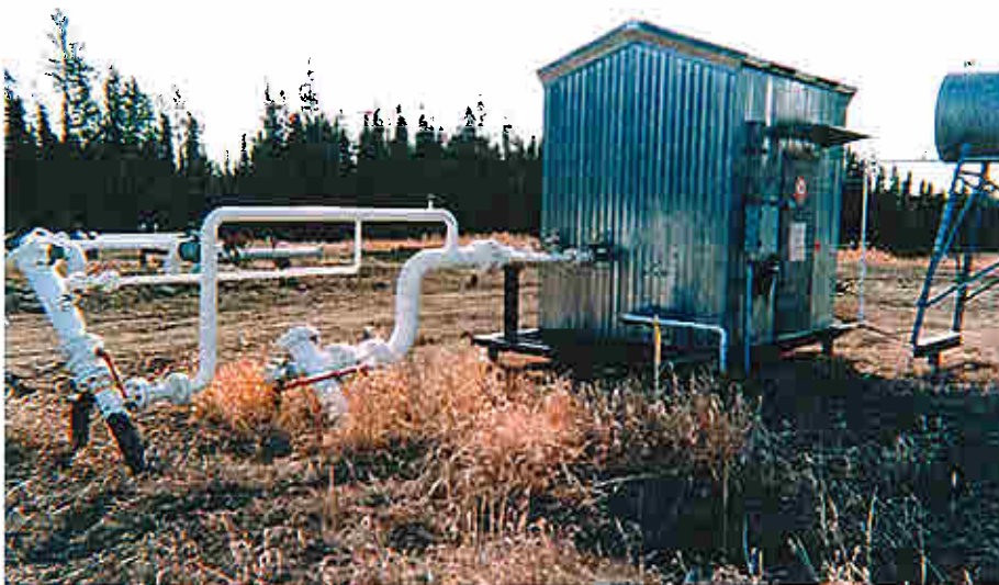
Gas wells are controlled by a metering skid in remote areas of N.W. Canada.
