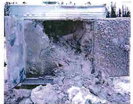
Catastrophic failures with V-Ball valves would fill the skids with sand.
