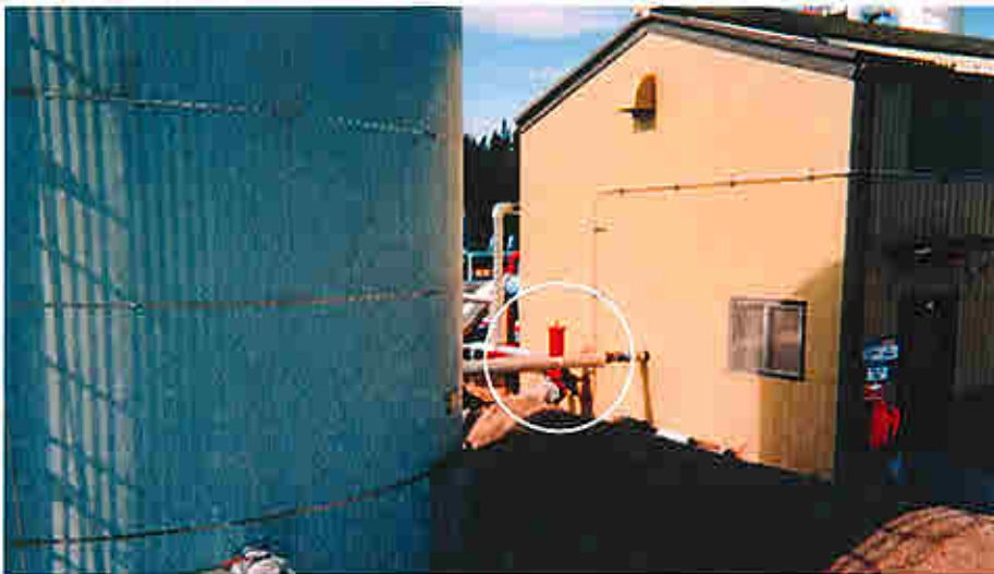
Inlet separator tank to remove water and sand from field gas. Series 5200 maintains level control.
